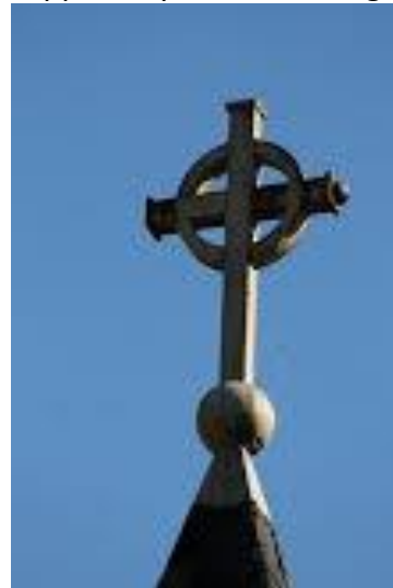
Repainting the cross on the steeple with funds supplied by Cliff and Marge Nix.
